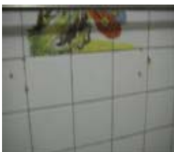
Fig. 15 No handrail in bathroom
