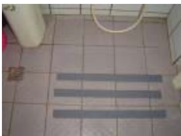
Fig. 19 Anti-slip in bathroom
